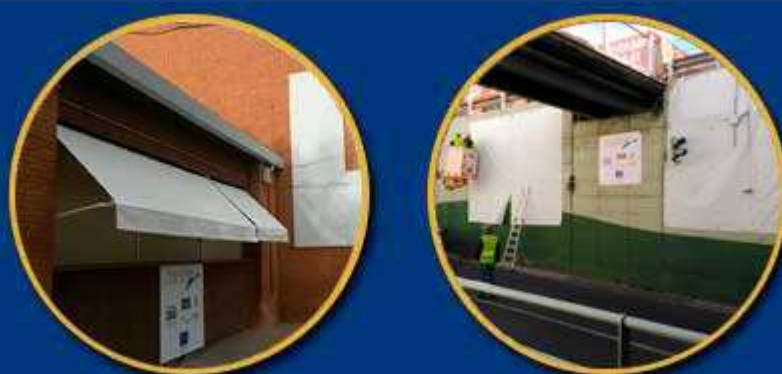
Photo A. Photocatalytic awning installed at the local school, with measuring and sampling systems
